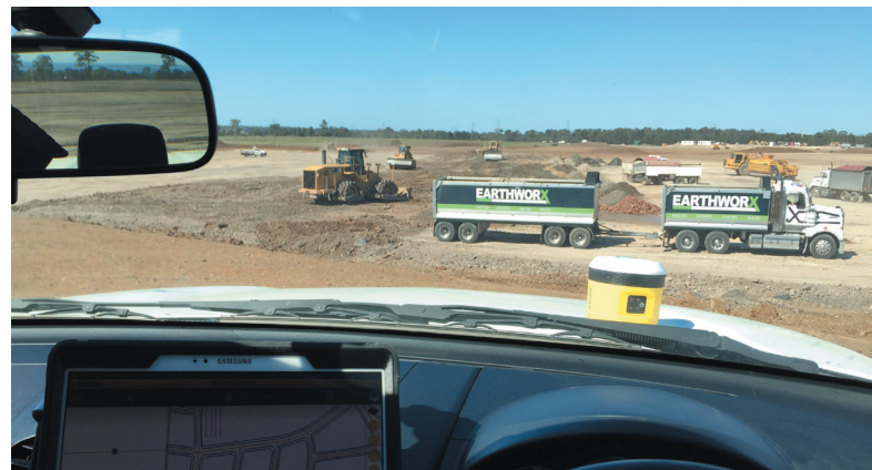
The Trimble SitePulse GNSS receiver sits on the vehicle’s bonnet, secured via a strong magnetic base. Inside the cab, the field manager and any passengers can view 3D digital site data on the field manager’s tablet device.
