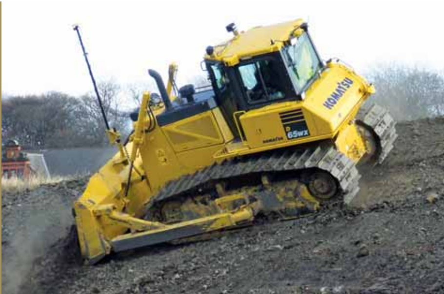
LEFT: Bulldozers were amongst the first machines to use GPS control technology
